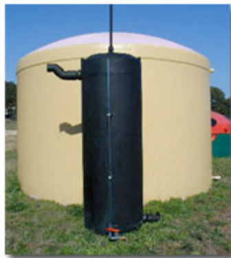
Tank with Eliminator UV lamp
